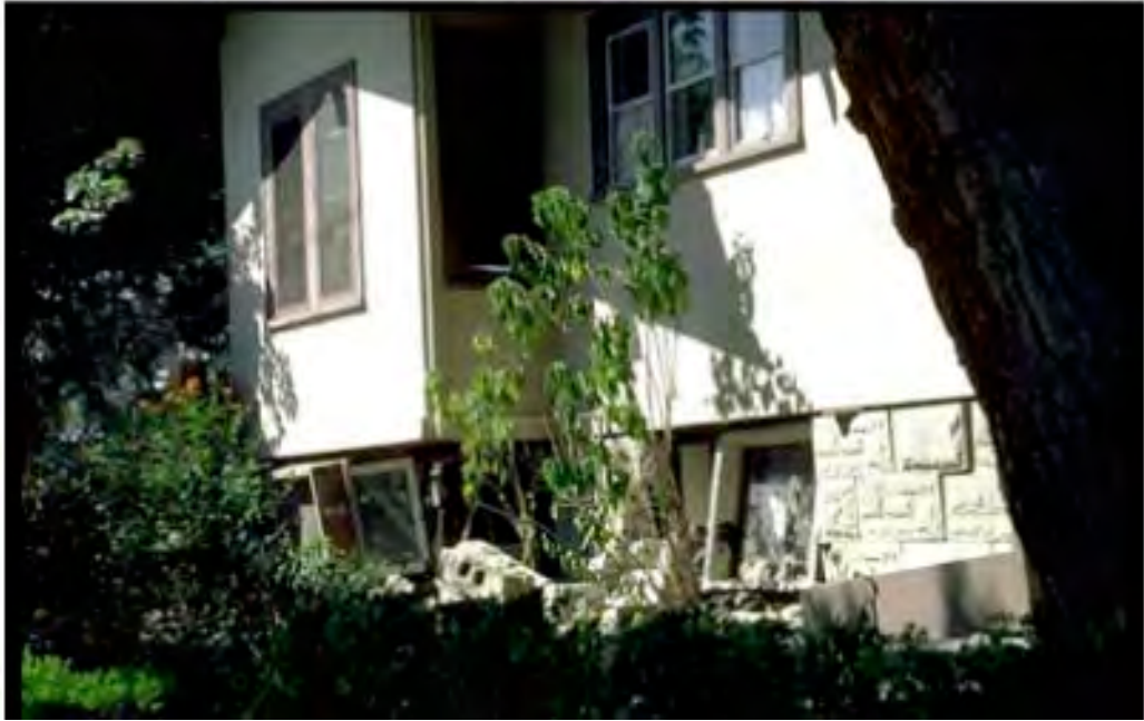
FIGURE 30.32 Hollow concrete-block foundation that failed during the magnitude 6.0 1987 Whittier, CA earthquake. (Photograph by Karl Steinbrugge and courtesy of the Steinbrugge Collection, Earthquake Engineering Research Center, University of California, Berkeley.)
