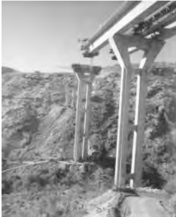
FIGURE 10.16a: Pine Valley Bridge, California. Construction state. (From California Department of Transportation. With permission.)
