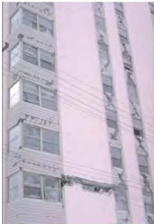
FIGURE 30.49 Damage to north side of Mt. McKinley Apartments. (Photograph by Karl Steinbrugge and courtesy of the Steinbrugge Collection, Earthquake Engineering Research Center, University of California, Berkeley.)
