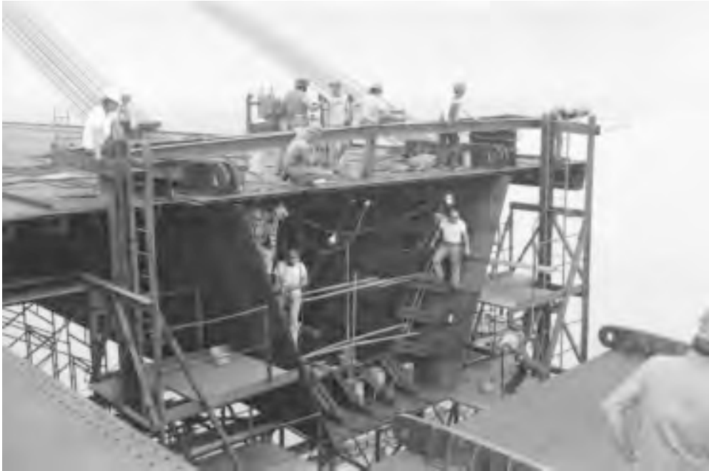
FIGURE 20.10: Luling Bridge deck steelwork erection, 1982; view looking northeast (refer to Figure 20.9) The twin box girders are 14 ft (4.3 m) deep; the deck plate is 7/16 in. (11 mm) thick. Girder section 16-east is being raised into position (lower right) and will be secured by large-pin hinge bars prior to fairing-up of joint holes and permanent bolting. Temporary erection stays are jumped forward as girder erection progresses.
