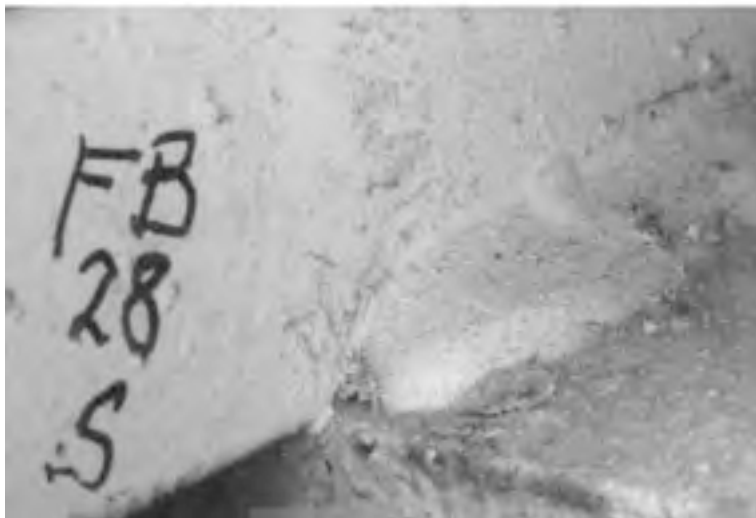
FIGURE 24.8: Fatigue crack originating from the upper weld toe of a fillet weld where the fillet weld terminates near the overlap of thick plates.
