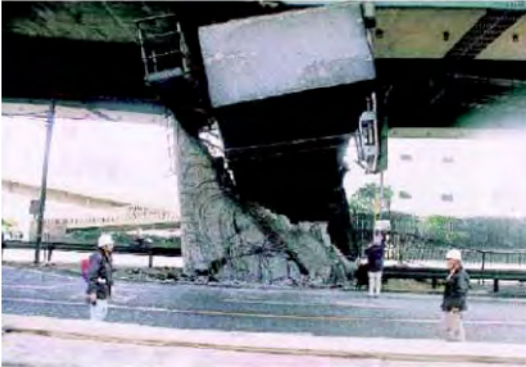
FIGURE 30.51 Shear failure of Pier 150 on Kobe Route 3.
