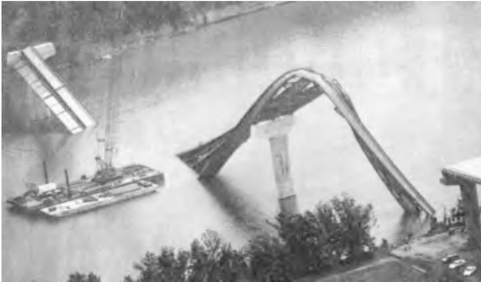
FIGURE 20.1: Failure of a steel girder bridge during erection, 1995. Steel bridge failures such as this one invite suspicion that the construction engineering aspects were not properly attended to.
