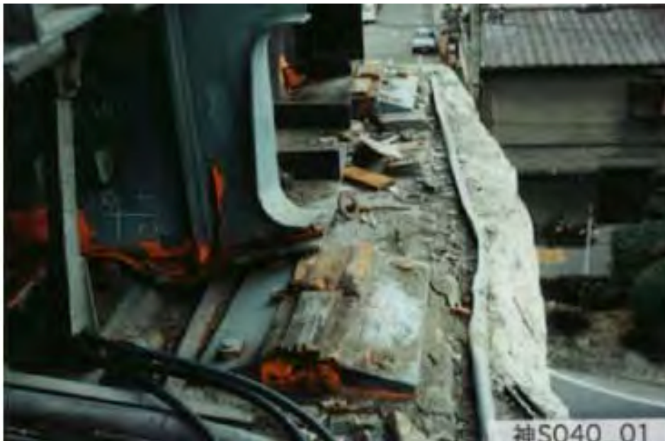
FIGURE 30.58 Broken bearings at Pier 40. (Courtesy of Hanshin Expressway Public Corporation.)
