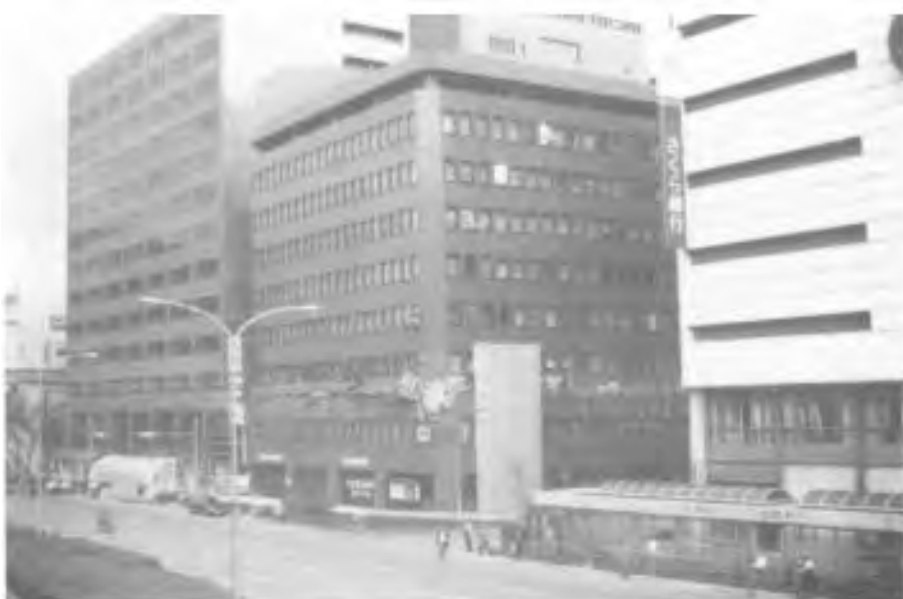
FIGURE 30.39 Ten-story steel and reinforced-concrete (SRC) building with third-floor collapse during the Kobe earthquake. (Courtesy of NIST [9].)
