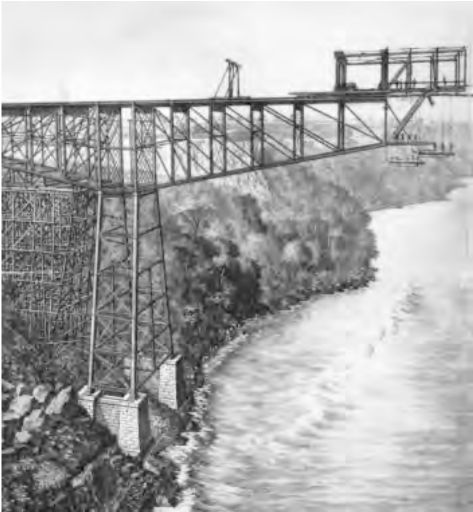
FIGURE 20.17: Niagara River railway cantilever truss bridge, near Niagara Falls, New York 1883. Massive wood erection traveler constructed side span on falsework, then cantilevered half of main span to midspan. Erection of other half of bridge was similar. First modern-type cantilever bridge, with 470-ft (143-m) clear main span having a 120-ft (37-m) center suspended span.
