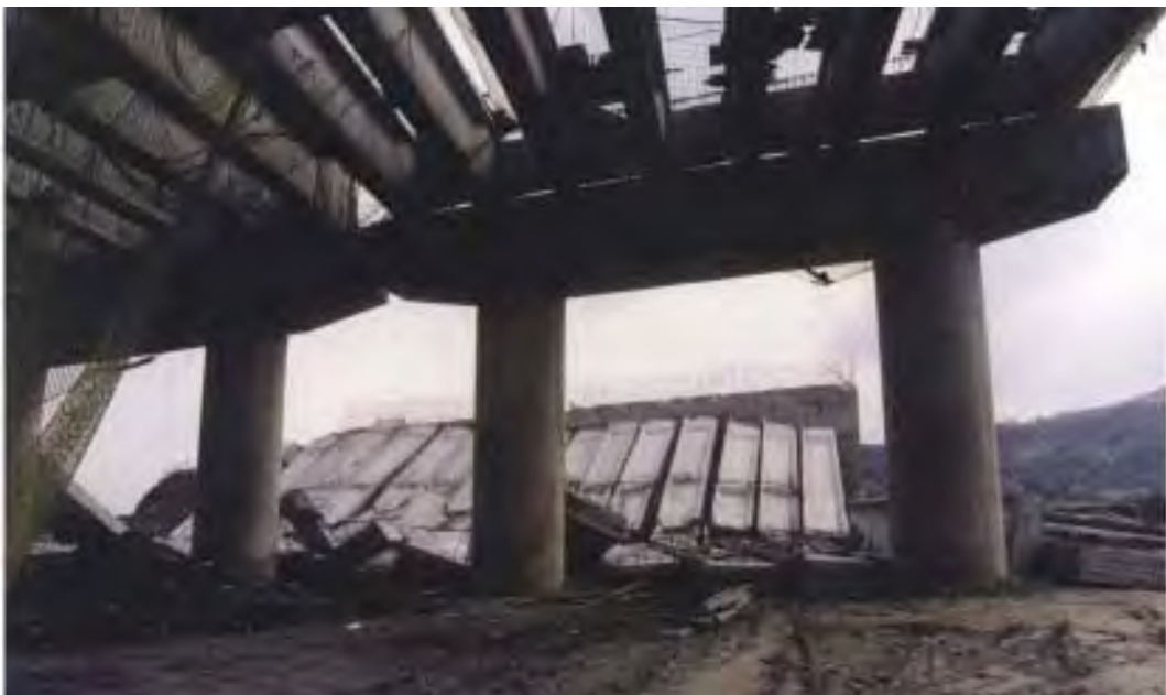
FIGURE 30.63 Precast, prestressed “I” girders during construction of new expressway in Taiwan that collapsed during the 1999 Ji Ji, Taiwan earthquake.
