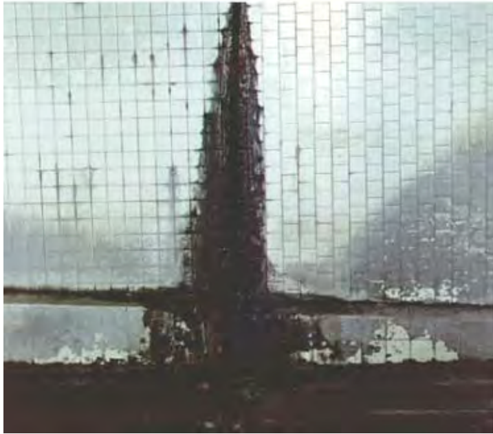
FIGURE 30.10 Liquefaction-induced damage to Webster Street Tube tunnel.
