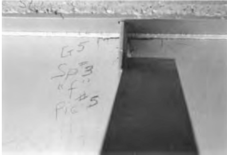
FIGURE 24.9: Typical distortion-induced cracking in the web gap of an attachment plate.
