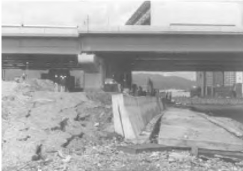
FIGURE 30.7 Liquefaction-caused bridge damage during Kobe earthquake.
