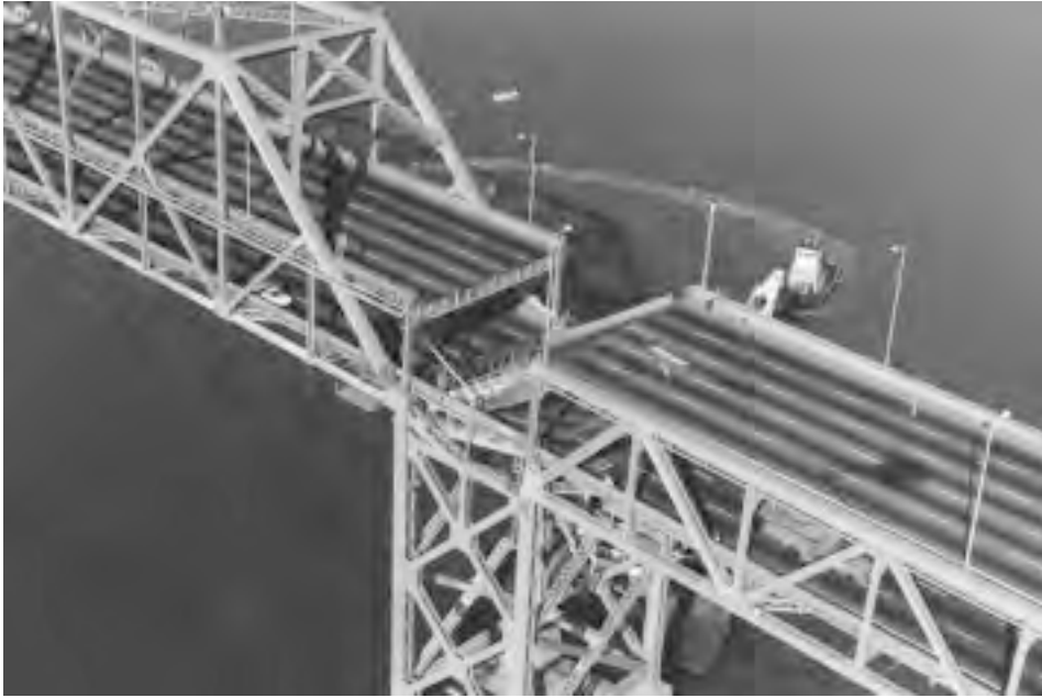
FIGURE 16.2: Aerial view of collapsed upper and lower decks of the San Francisco-Oakland Bay Bridge (I-80) following the 1989 Loma Prieta earthquake in California. (Photo by California Department of Transportation. With permission.)
