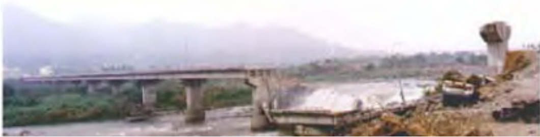
FIGURE 30.67 The Dajia River Bridge and 6-m fault scarp.
