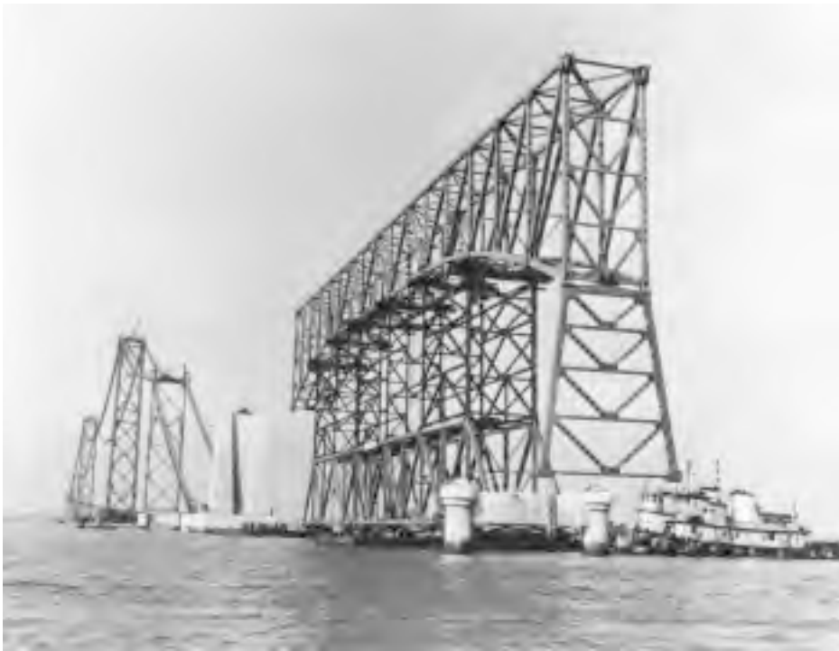
FIGURE 20.31: Floating-in erection of a truss span, first Chesapeake Bay Bridge, Maryland, 1952. A 480-ft (146-m) truss span, weighing 850 tons, supported on falsework consisting of a permanent deck-truss span along with temporary members, is being floated-in for landing onto its piers. Suspension bridge cables are under construction in background. (Courtesy of Bethlehem Steel Corporation.)
