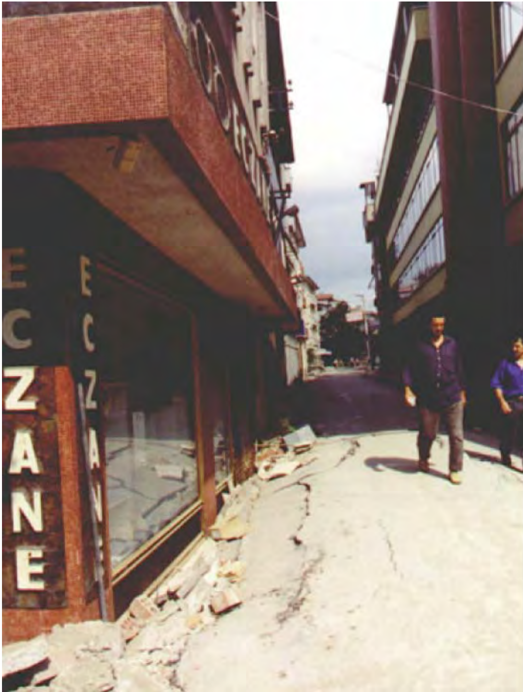
FIGURE 30.6 Settlement of building due to loss of bearing during the 1999 Kocaeli earthquake.
