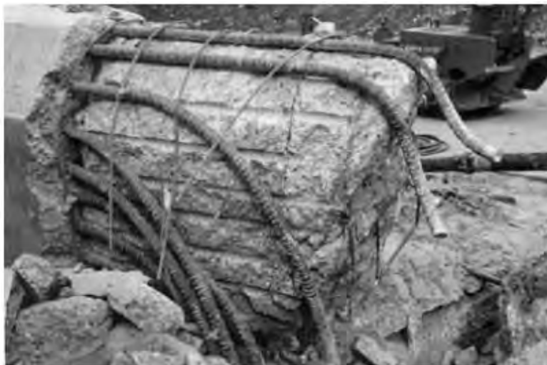
FIGURE 30.36 Failure of connection of column to footing.
