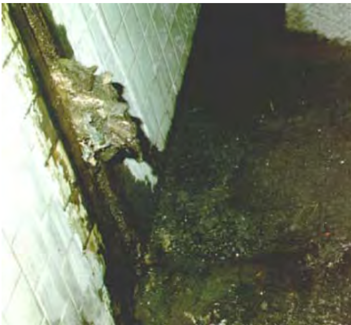
FIGURE 30.11 Liquefaction-induced damage to Webster Street Tube tunnel.
