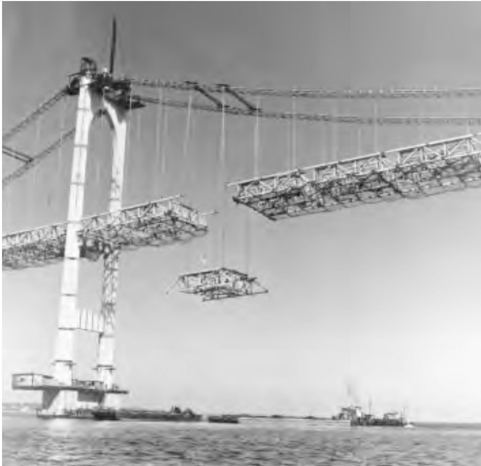
FIGURE 20.40: Suspended deck steelwork erection, the Newport Bridge suspension spans, Narragansett Bay, R.I., 1968. The closing mainspan deck section is being raised into position by two cable travelers, each made up of a pair of 36-in. (0.91-m) wide-flange rolled beams that ride the cables on wooden wheels. The closing section is 40-1/2 ft (12 m) long at top-chord level, 66 ft (20 m) wide and 16 ft (5 m) deep, and weighs about 140 tons. (Courtesy of Bethlehem Steel Corporation.)
