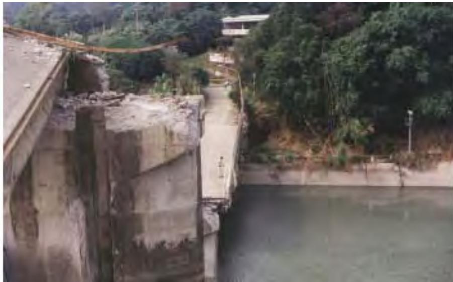
FIGURE 30.65 North end of Shih Kang Dam after the Ji Ji, Taiwan earthquake.
