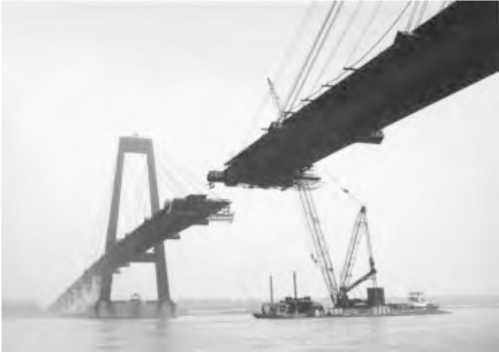
FIGURE 20.9: Cable-stayed orthotropic-steel-deck bridge over Mississippi River at Luling, La., 1982; view looking northeast. The main span is 1222 ft (372 m); the A-frame towers are 350 ft (107 m) high. A barge-mounted ringer derrick erected the main steelwork, using a 340-ft (104-m) boom with a 120-ft (37-m) jib to erect tower components weighing up to 183 tons, and using a shorter boom for deck components. Cable stays at the ends of projecting cross girders are permanent; others are temporary erection stays. Girder section 16-west of north portion of bridge, erected a few days previously, is projecting at left; companion girder section 16-east is on barge ready for erection (see Figure 20.10).
