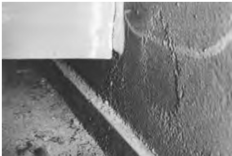
FIGURE 24.7: Cracking through the throat of fillet welds on an attachment plate.
