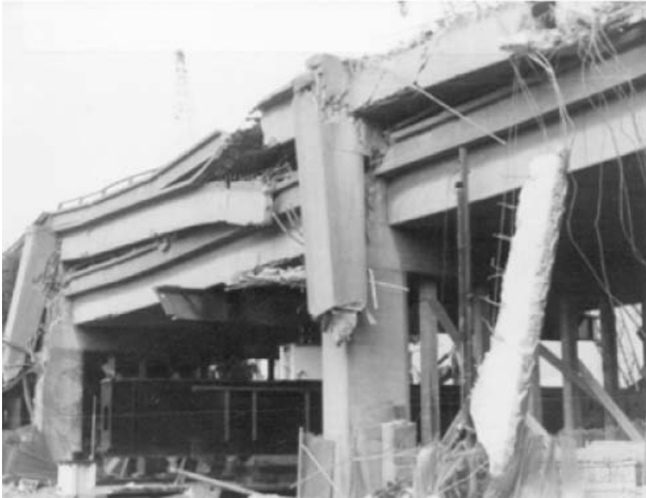
FIGURE 30.28 Damage to Cypress Street viaduct.
