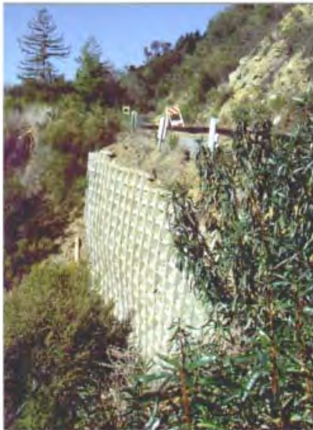
FIGURE 30.74 Crib wall continues to support steeply sloping soil in Santa Cruz after the 1989 Loma Prieta earthquake. (Courtesy of the Earthquake Engineering Research Institute; photograph by Marshall Lew [1a].)
