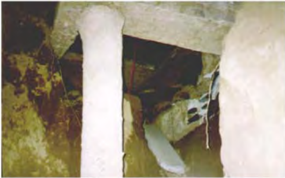
FIGURE 30.69 Washed-out abutment fill caused by a water pipe break.
