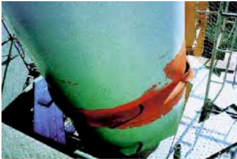
FIGURE 30.55 Torn buckle of steel column on Route 3 after the 1995 Kobe earthquake. (Courtesy of Hanshin Expressway Public Corporation.)
