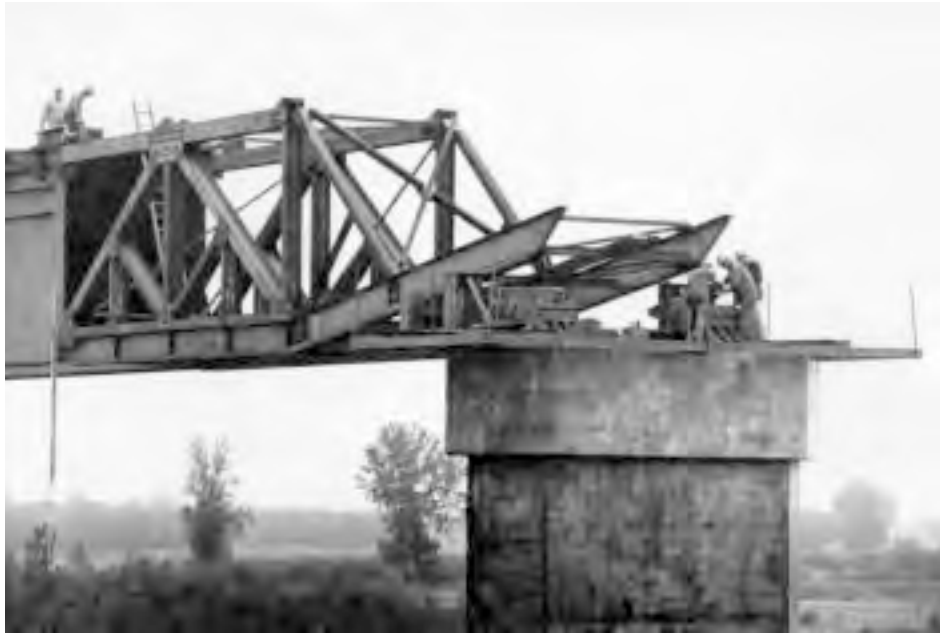
Figure 20.41b Launching nose rides up onto pier 5 skidway units, removing girder-train leading-end sag.
