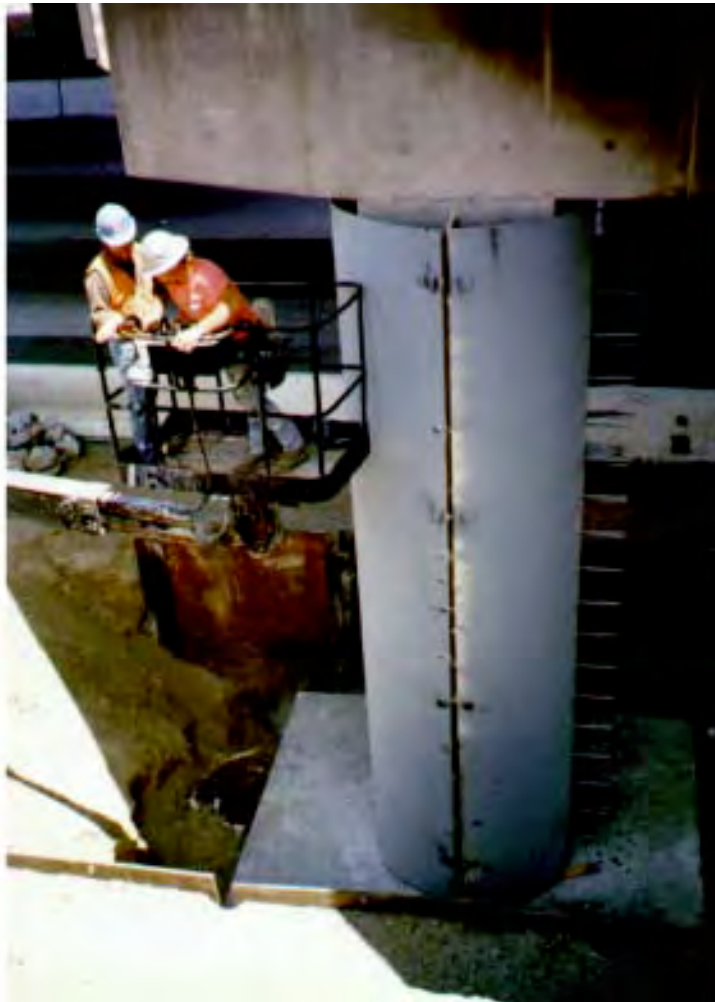
FIGURE 30.89 Steel shell being wrapped around a concrete bridge column to increase its ductility and shear strength.
