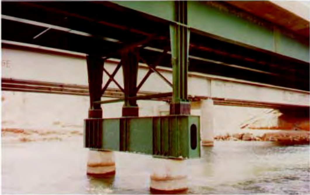
FIGURE 30.86 Lead–rubber isolation bearings on the All American Canal Bridge in California.
