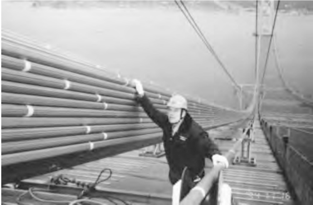
FIGURE 20.46: Parallel-wire-strand main cable, Akashi Kaikyo suspension bridge, Kobe, Japan, 1994. The main span is 6529 ft (1990 m), by far the world's longest. The PWS at right is being towed across the spans, supported on rollers. The completed cable is made up of 290 PWS, making a total of 36,830 wires, and has a diameter of 44.2 in. (1122 mm) following compaction—the largest bridge cables built to date. Each 127-wire PWS is about 2-3/8 in. (60 mm) in diameter. (Courtesy of Nippon Steel—Kobe Steel.)
