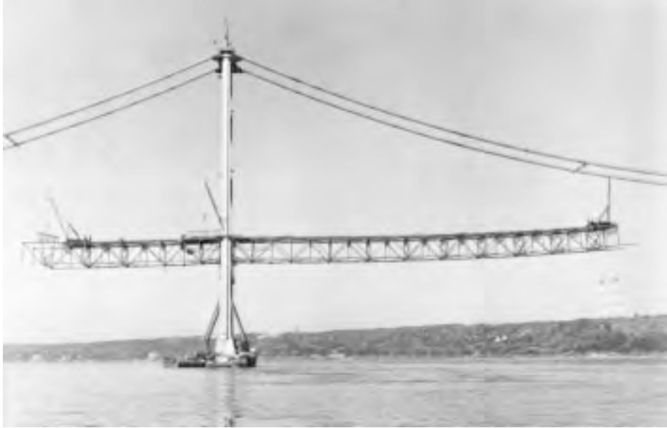
FIGURE 20.27: Erection of suspended deck steelwork, second Tacoma Narrows Bridge, Washington, 1950. The Chicago boom on the tower raises deck steelwork components to deck level, where they are transported to deck travelers by material cars. Each truss double panel is connected at top-chord level to previously erected trusses, and left open at bottom-chord level to permit temporary upward deck curvature, which results from the partial loading condition of the main suspension cables. The main span (at right) is 2800 ft (853 m), and side spans are 1100 ft (335 m). The stiffening trusses are 33 ft (10 m) deep and 60 ft (18 m) on centers. Tower-base kneebraces (see Figure 20.24) show clearly here.
