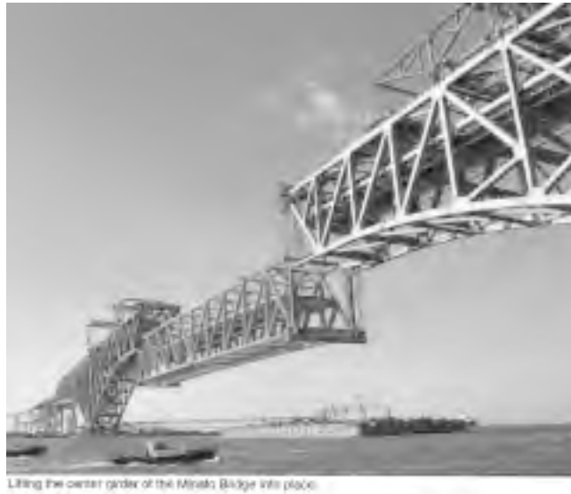
FIGURE 10.43: Lifting erection of the Minato Oh-Hashi, Japan. (Gerber bridge, 1974). (From Hanshin Expressway Public Corporation, Techno Gallery , Osaka, Japan, 1994. With permission.)
