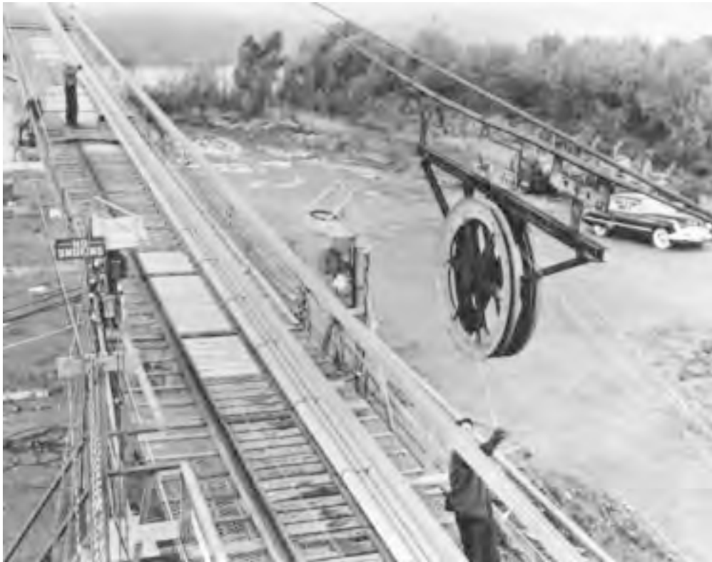
Figure 20.25a Tramway starts across from east anchorage carrying two wire loops. Three 460-wire strands have been spun, with two more under construction. Tramway spinning wheels pull wire loops across the three spans from east anchorage to west anchorage. Suspended footbridges provide access to cables. Spinning goes on 24 hours per day.
