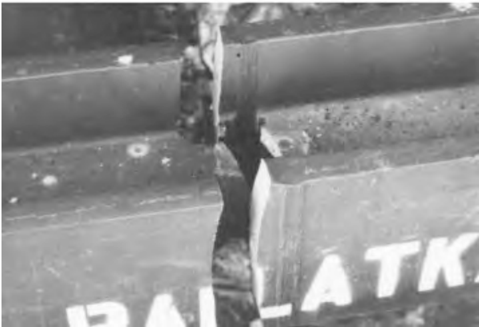
FIGURE 24.4: (a) View of jumbo section used as tension chord in a roof truss and (b) closeup view of fracture in web originating from weld access holes at welded splice.
