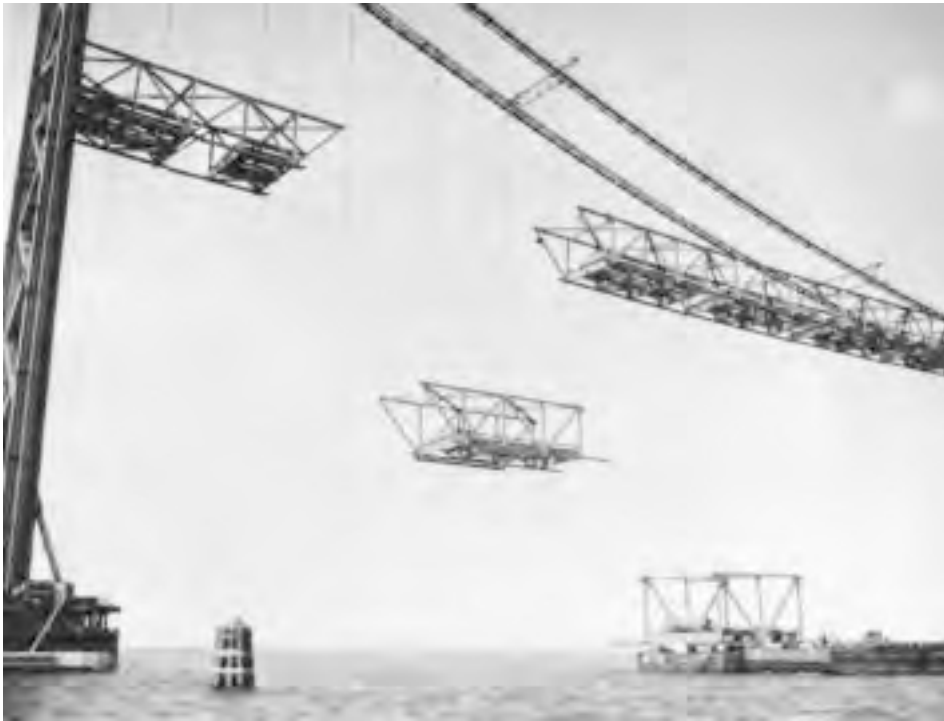
FIGURE 20.33: Erection of suspension bridge deck structure, first Chesapeake Bay Bridge, Maryland, 1952. A typical four-panel through-truss deck section, weighing 99 tons, has been picked from the barge and is being raised into position using four sets of lifting falls attached to main suspension cables. The closing deck section is on the barge, ready to go up next. (Courtesy of Bethlehem Steel Corporation.)
