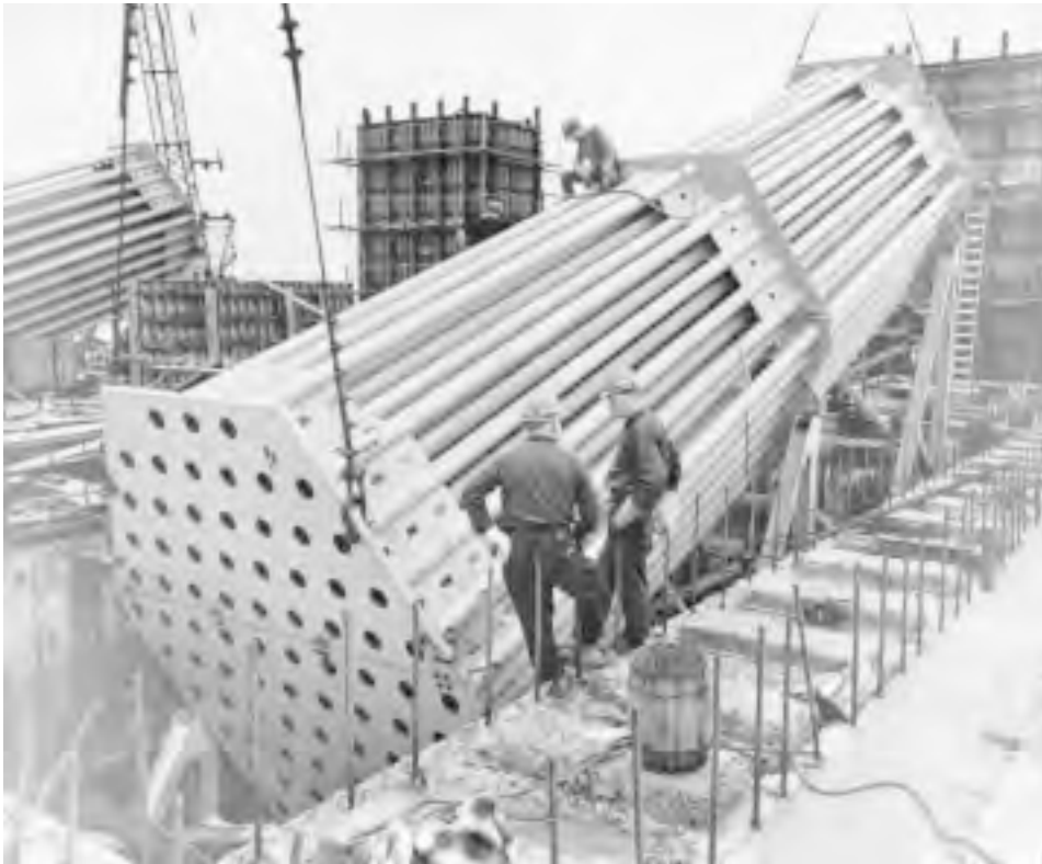
FIGURE 20.38: Pipe-type anchorage for parallel-wire-strand (PWS) cables, the Newport Bridge suspension spans, Narragansett Bay, R.I., 1967. Pipe anchorages shown will be embedded in anchorage concrete. The socketed end of each PWS is pulled down its pipe from the upper end, then seated and shim-adjusted against the heavy bearing plate at the lower end. The pipe-type anchorage is much simpler and less costly than the standard anchor-bar type used with aerial-spun parallel-wire cables (see Figure 20.25b). (Courtesy of Bethlehem Steel Corporation.)
