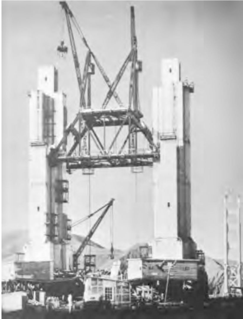
FIGURE 20.22: Erecting south tower of Golden Gate Bridge, San Francisco, 1935. A creeper traveler with two 90-ft (27-m) booms erects a tier of tower cells for each leg, then is jumped to the top of that tier and proceeds to erect the next tier. The tower legs are 90 ft (27 m) center-to-center and 690 ft (210 m) high. When the traveler completed the north tower (in background) it erected a Chicago boom on the west tower leg, which dismantled the creeper, erected tower-top bracing, and erected two small derricks (one shown) to service cable erection. Each tower contains 22,200 tons of steelwork.
