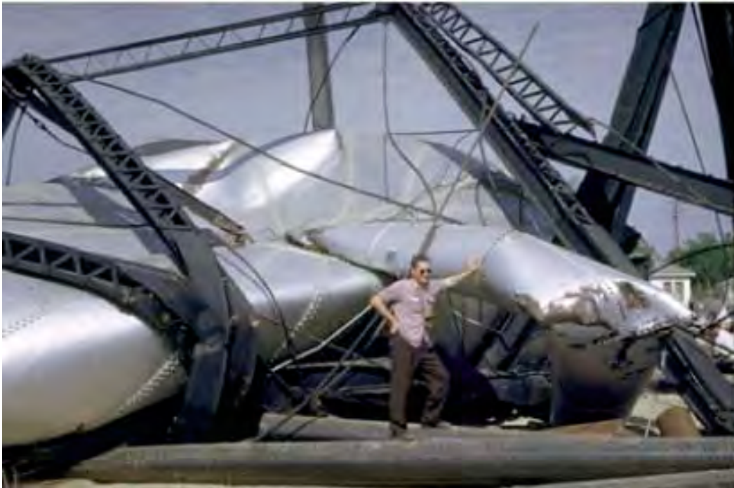
FIGURE 30.62 California Water Service 150,000-gallon tank on six legs (Bakersfield, CA). The typical failure of tanks is upside down, with riser on top. Photograph taken July 25, 1952, after the July 21, 1952, Kern County, CA earthquake (magnitude 7.69). (Photograph by Karl Steinbrugge and courtesy of the Steinbrugge Collection, Earthquake Engineering Research Center, University of California, Berkeley.)
