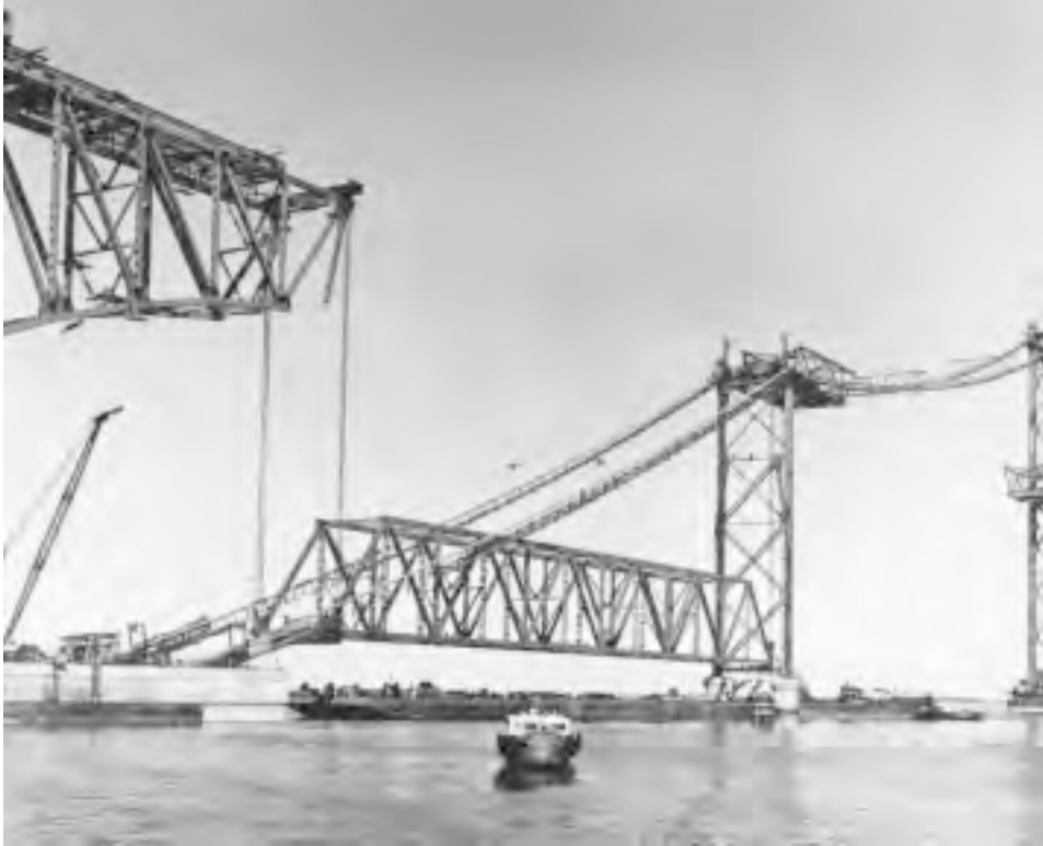
FIGURE 20.32: Erection of a truss span by hoisting, first Chesapeake Bay Bridge, Maryland, 1952. A 360-ft (110-m) truss span is floated into position on barges and picked clear using four sets of lifting falls. Suspension bridge deck is under construction at right. (Courtesy of Bethlehem Steel Corporation.)
