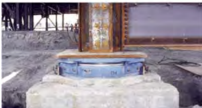
FIGURE 30.79 One of the 267 friction pendulum devices for the new San Francisco Airport International Terminal. (Courtesy of Earthquake Protection Systems, Inc.)
