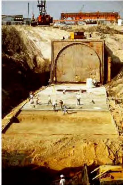
FIGURE 15B.7 Second downtown Elizabeth River Tunnel, VA. (©1983 Parsons Brinckerhoff, Inc. With permission.)
