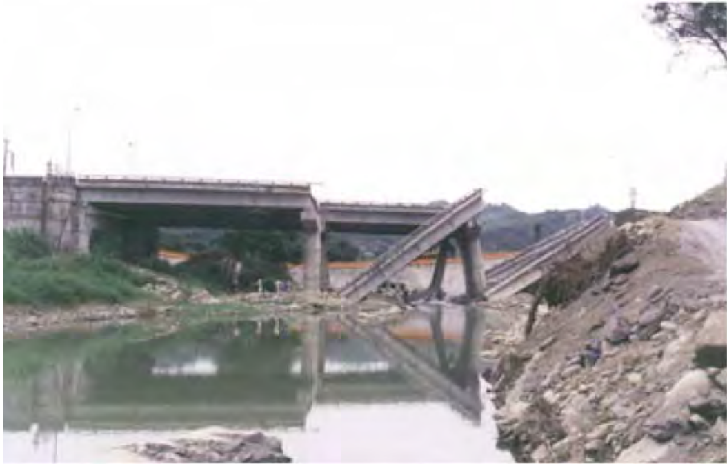
FIGURE 30.19 Collapse of Tsu Wei Bridge due to landslide during the Ji Ji, Taiwan earthquake.
