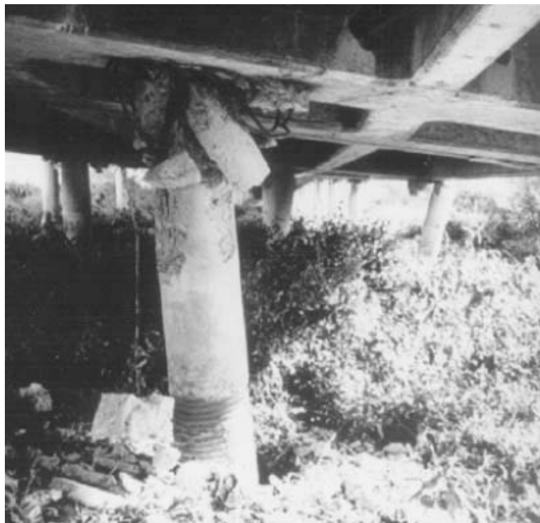
FIGURE 30.25 Broken piles under the bridge.
