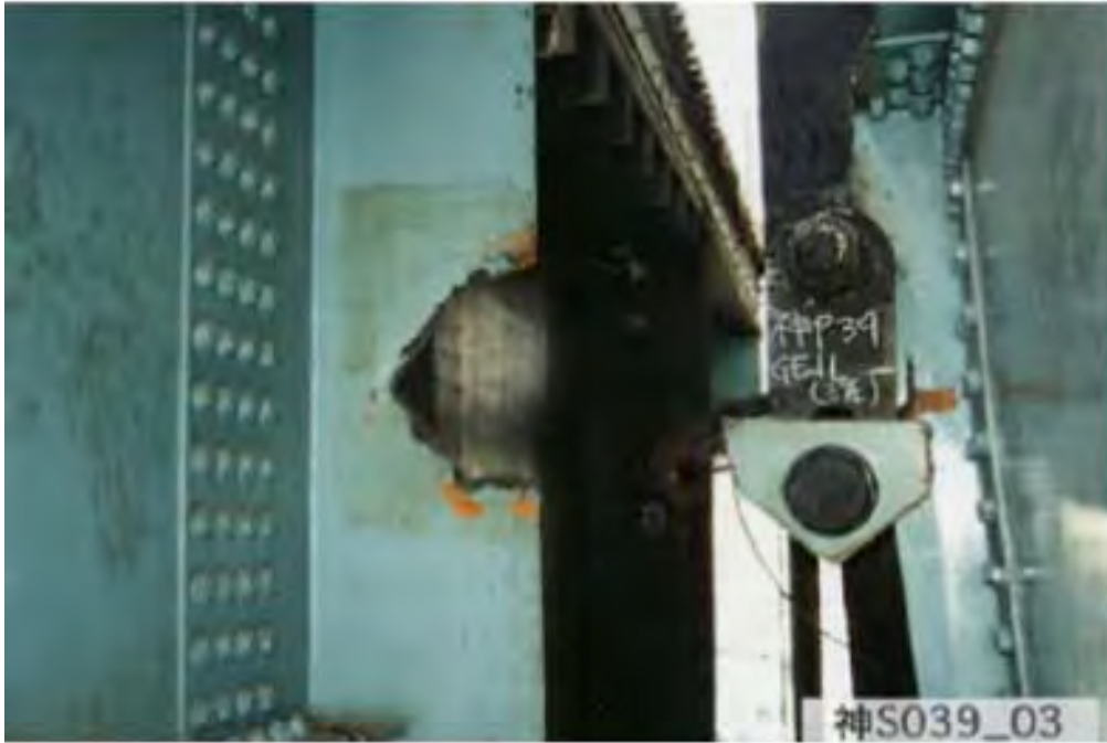
FIGURE 30.57 Broken restrainer at Pier 39. (Courtesy of Hanshin Expressway Public Corporation.)
