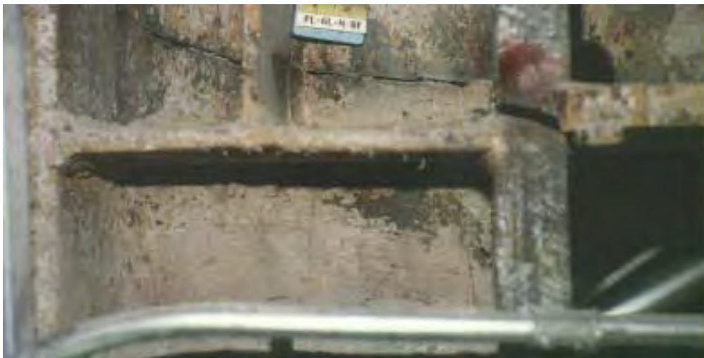
FIGURE 30.60 Steel moment-resisting frame connection after the 1994 Northridge earthquake. (From EQE International, Inc., Steel's performance in the Northridge earthquake, EQE International Fall Review , p. 1, 1994. With permission.)
