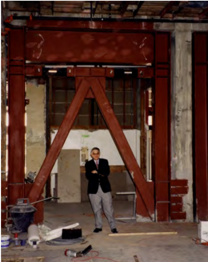
FIGURE 30.83 The steel frames included fluid viscous dampers to reduce story drift. (Courtesy of Marr-Shaffer & Miyamoto, Structural Engineers.)
