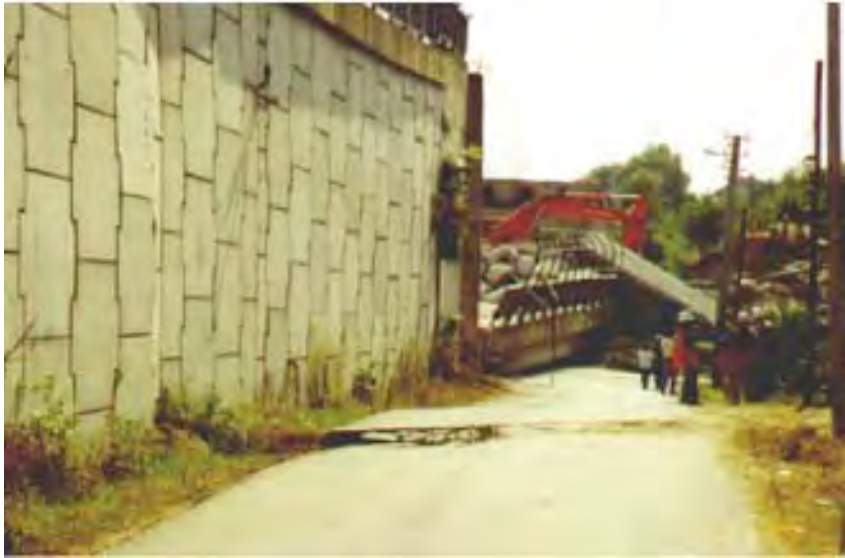
FIGURE 30.73 Mechanically stabilized earth (MSE) wall continues to support the embankment behind the collapsed Arifiye Overcrossing after the 1999 Kocaeli, Turkey, earthquake.
