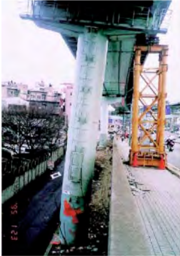
FIGURE 30.54 Pier 585 on Kobe Route 3 during the 1995 Kobe earthquake. (Courtesy of Hanshin Expressway Public Corporation.)
