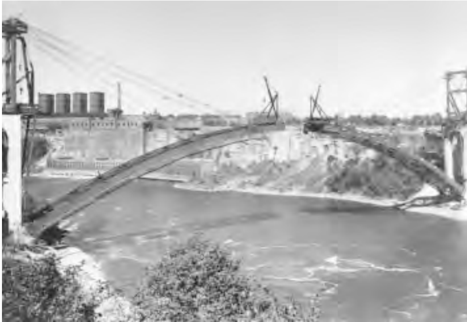
FIGURE 20.2: Erection of arch ribs, Rainbow Bridge, Niagara Falls, New York, 1941. Bridge span is 950 ft (290 m), with rise of 150 ft (46 m); box ribs are 3 \times 12 ft ( 0.91 \times 3.66 m). Tiebacks were attached starting at the end of the third tier and jumped forward as erection progressed (see Figure 20.3). Much permanent steelwork was used in tieback bents. Derricks on approaches load steelwork on material cars that travel up arch ribs. Travelers are shown erecting last full-length arch-rib sections, leaving only the short, closing crown sections to be erected. Canada is at right, the U.S. at left. (Courtesy of Bethlehem Steel Corporation.)
