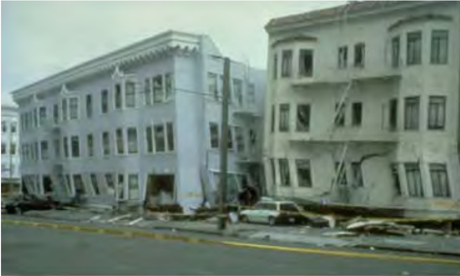
FIGURE 30.37 Soft-story collapse in San Francisco during the 1989 Loma Prieta earthquake. (Courtesy of the U.S. Geological Service [10].)
