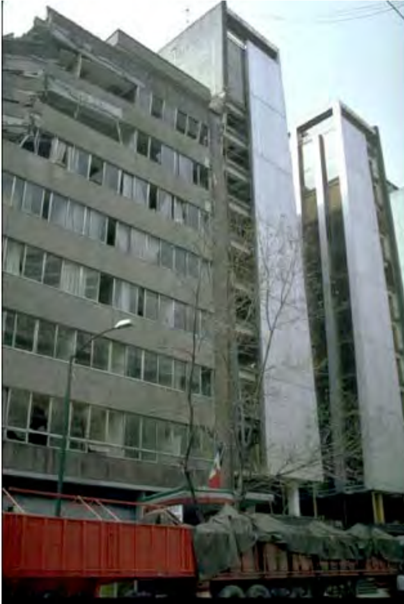
FIGURE 30.31 Damaged 10-story building between the Plaza de la Constitution and Zona Rosa in Mexico City. (Photograph by Karl Steinbrugge and courtesy of the Steinbrugge Collection, Earthquake Engineering Research Center, University of California, Berkeley.)
