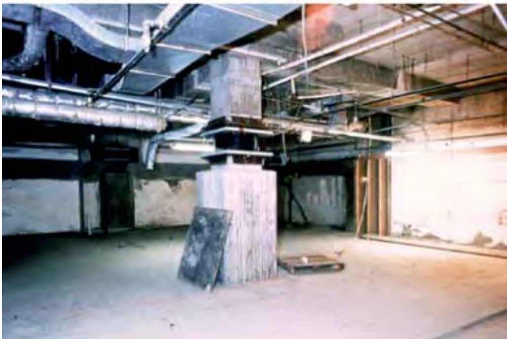
FIGURE 30.85 Concrete columns at Long Beach VA Hospital that were cut at mid-height and installed with lead–rubber isolation devices. (Courtesy of Dynamic Isolation Systems, Inc.)
