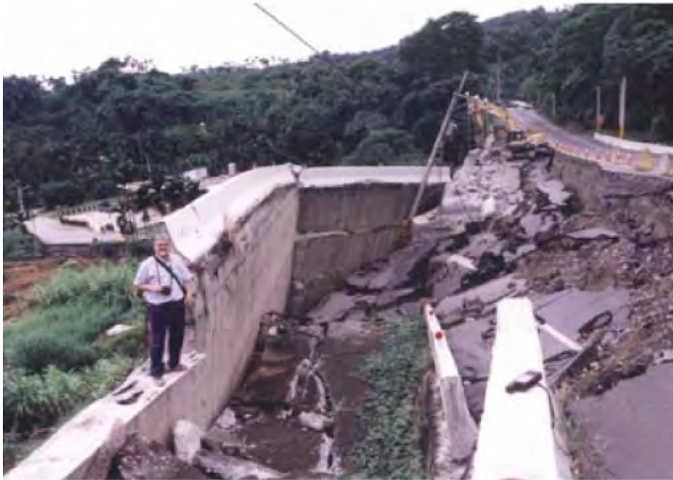
FIGURE 30.13 Gravity retaining wall pushed outward by landslide.
