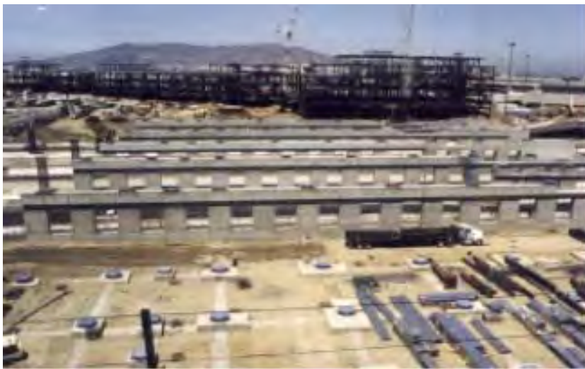
FIGURE 30.78 Layout of foundations and friction pendulum devices for the new San Francisco Airport International Terminal. (Courtesy of Earthquake Protection Systems, Inc.)
