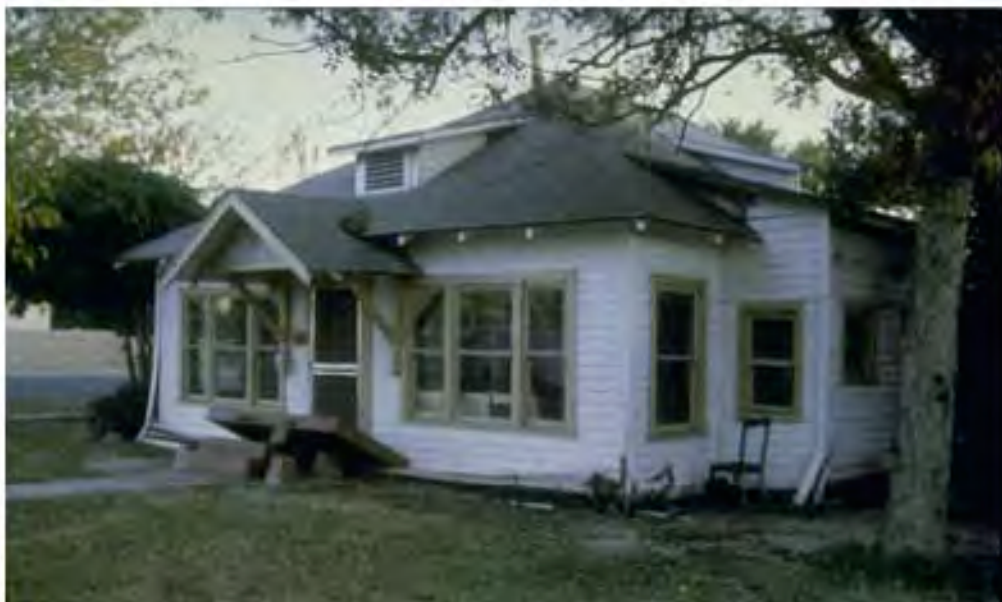
FIGURE 30.34 House that fell from its foundation during the 1971 San Fernando earthquake. (Courtesy of Steinbrugge Collection, Earthquake Engineering Research Center, University of California, Berkeley.)
