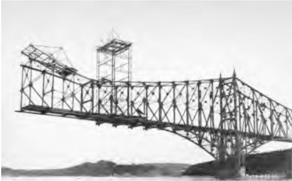
FIGURE 20.11: First Quebec railway cantilever bridge, 23 August 1907. Cantilever erection of south main span, 6 days before collapse. The tower traveler erected the anchor span (on falsework) and then the cantilever arm; then erected the top-chord traveler, which is shown erecting suspended span at end of cantilever arm. The main span of 1800 ft (549 m) was the world's longest of any type. The sidespan bottom chords second from pier (arrow) failed in compression because latticing connecting chord corner angles was deficient under secondary bending conditions.
