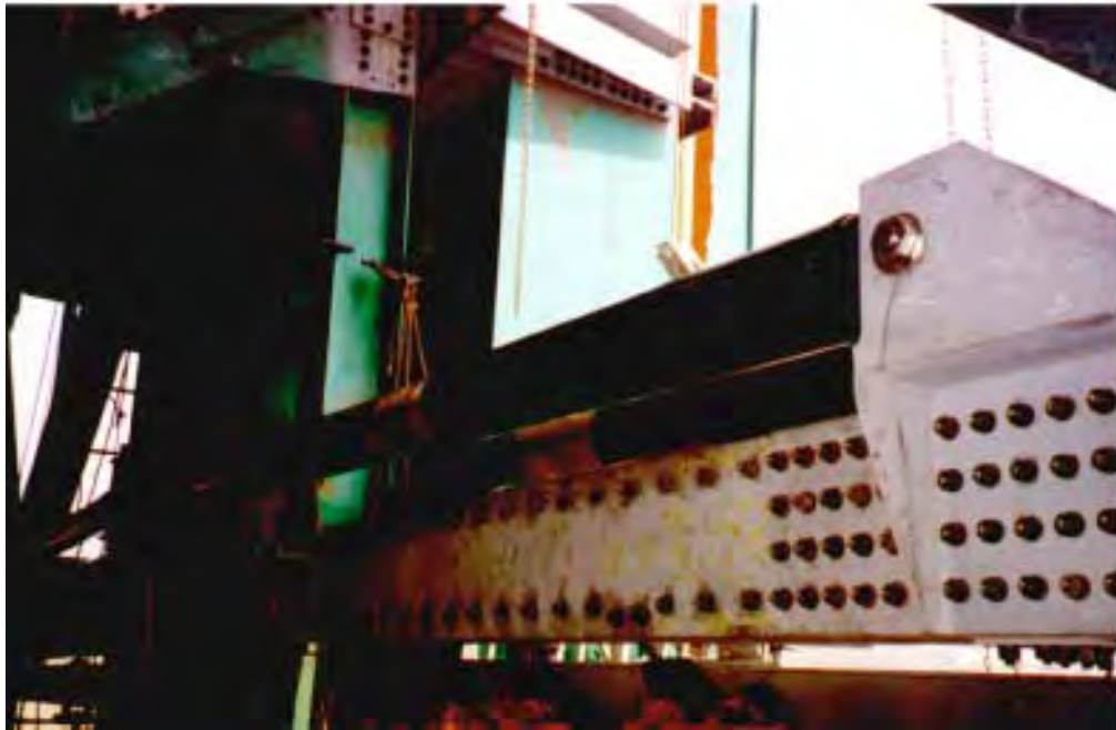
FIGURE 30.88 The Vincent Thomas Bridge retrofit that provided gaps between the decks and the towers and also fluid viscous dampers to dissipate energy. (Courtesy of Enidine, Inc.)
