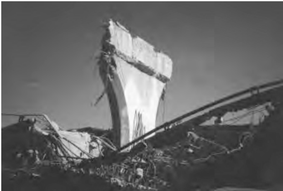
FIGURE 16.4: Collapsed SR-14/I-5 south connector overhead following the 1994 Northridge earthquake in California. (Photo by James MacIntyre. With permission.)
