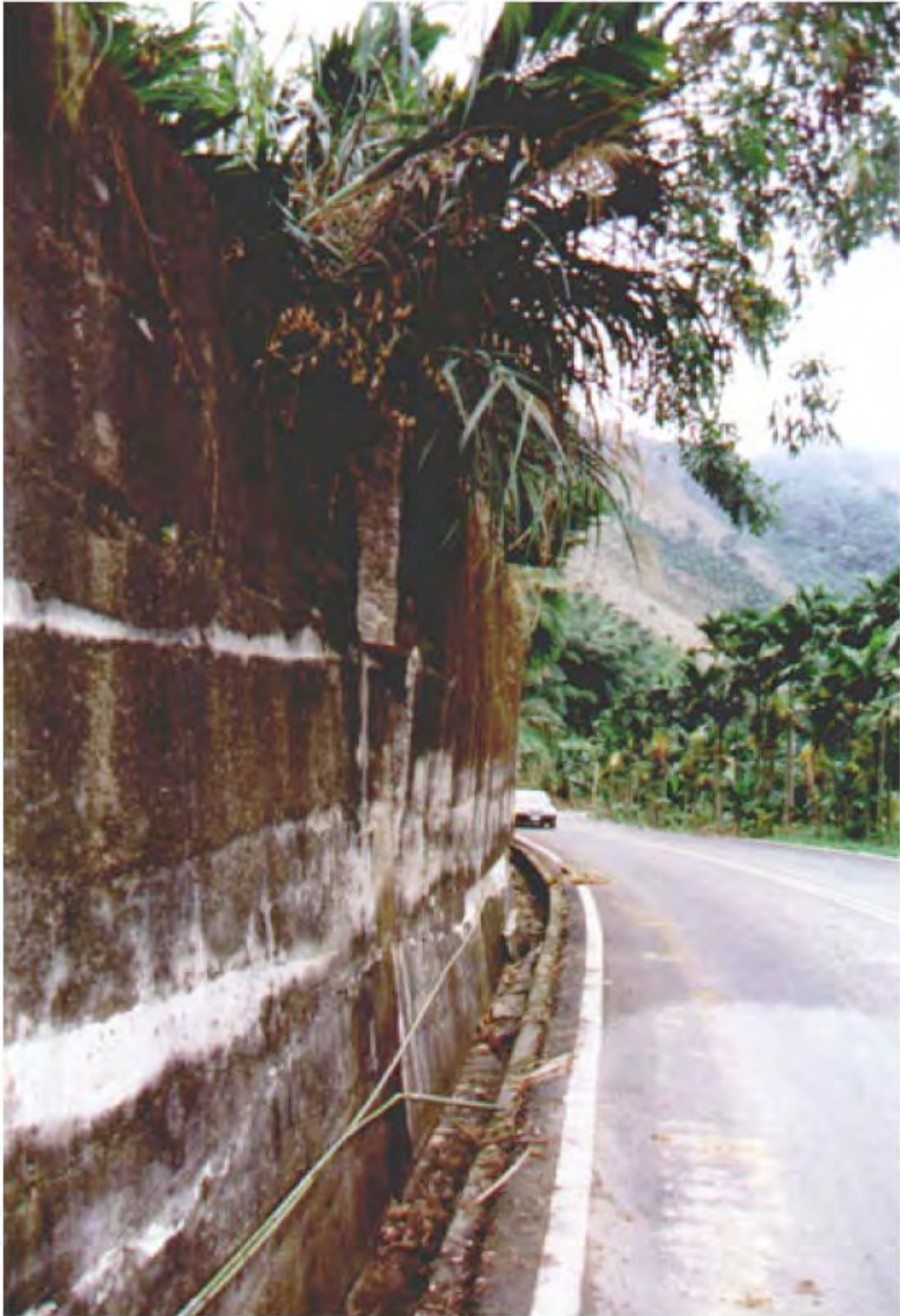
FIGURE 30.14 Gravity retaining wall with shear damage from landslide.
